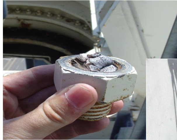
Case b, crack in bolt (FAT 50)
